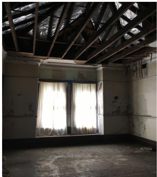
PICTURE 30 – INTERNAL VIEW SHOWING DILAPIDATED CEILING.
