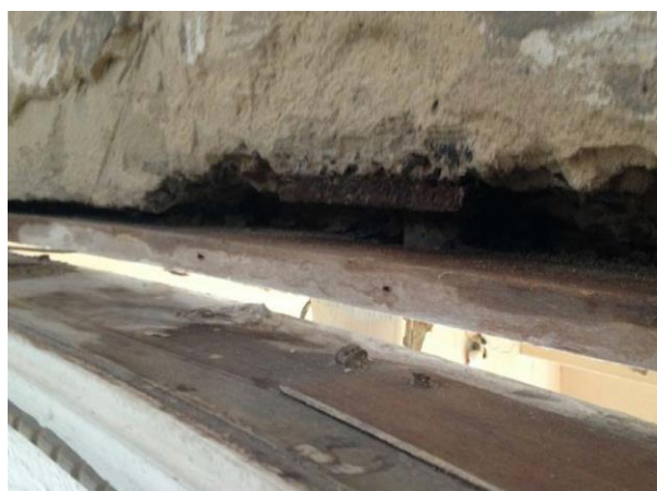
PICTURE 42 – DETAIL SHOWING CONCRETE CANCER
